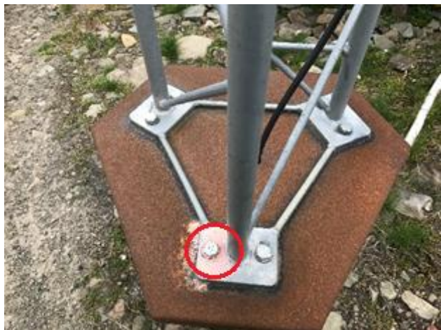
Figure 35. Circle points out the bolt, which was used for survey at the Reference point in Svea.
