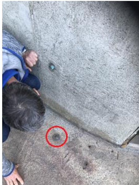
Figure 22. Circle points to the reference point at the entrance into the pipe of power plant in Longyearbyen. This point was used in the survey (LRP1).
