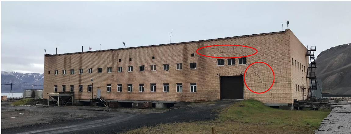
Figure 18. Cracks (highlighted with red circles) on the north-facing wall of the multi-purpose garage in Pyramiden.
