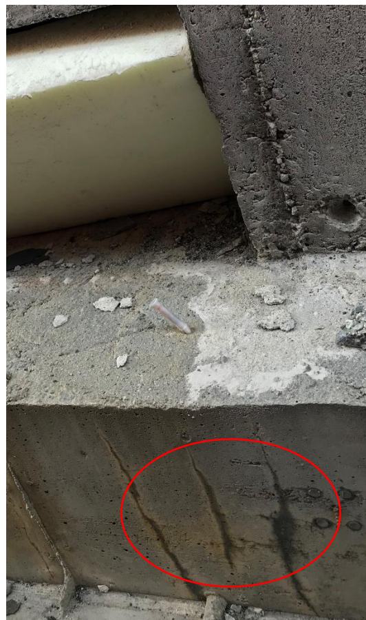
Figure 23. Cracks (highlighted with red circles) on foundation of the “Magnetittlageret” garage.
