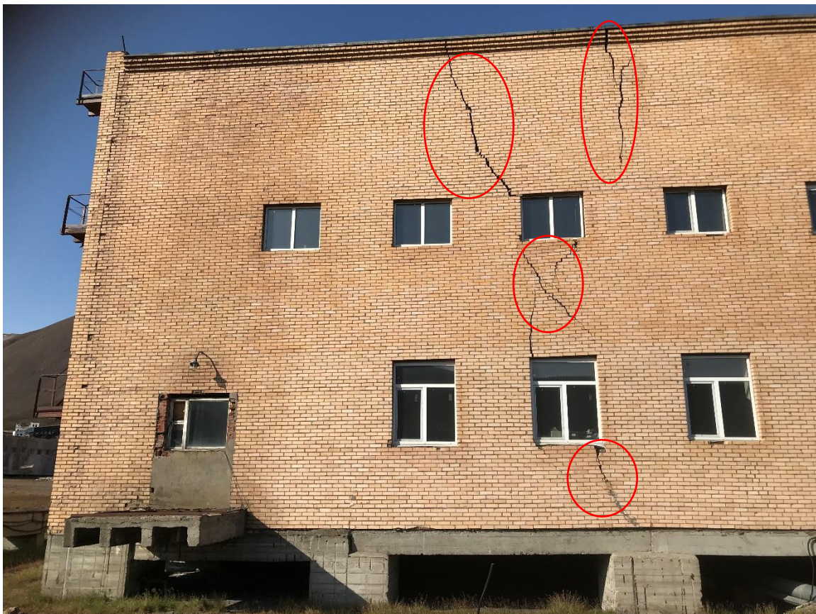
Figure 19. Cracks (highlighted with red circles) on the south-facing wall of the multi-purpose garage in Pyramiden.
