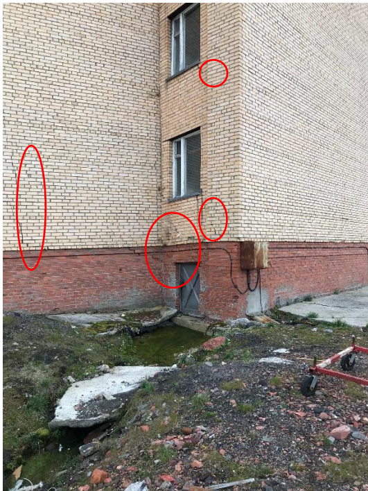
Figure 16. Drainage coming from under the building "Komplex GRZ" in Barentsburg and cracks (highlighted with red circles).
